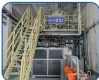
Zone of rectification
